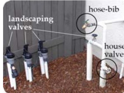
Photo 1 - Hose bib and piping
