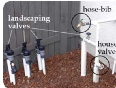
Photo 1 - Hose bib and piping
