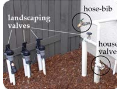
Photo 1 - Hose bib and piping
